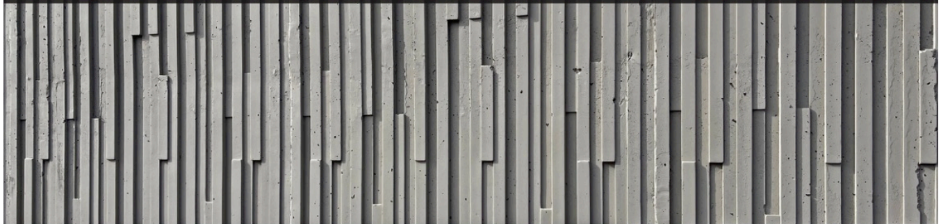
WSDOT Standard Patterning Above / 10'-12' Tall Wall Shown Below Creates a Dead Space
